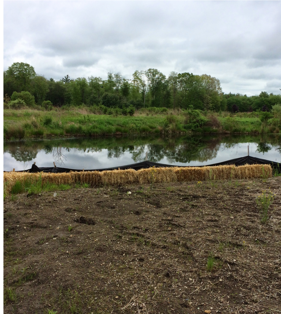
Erosion control measures along a wetland (Wilson 2023)
